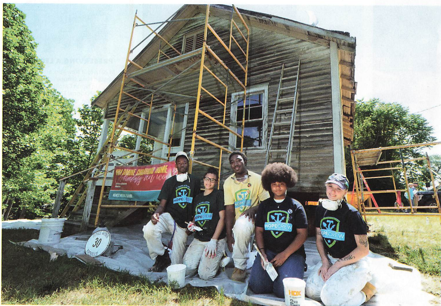
ABOVE: Members of the Hands-On Preservation Experience (HOPE) Crew, which trains youth in historic-preservation techniques, helping to restore the home's facade last summer.
